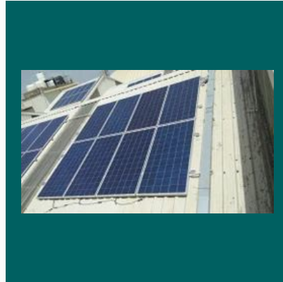
Tin Shade Solar Panel Structure
