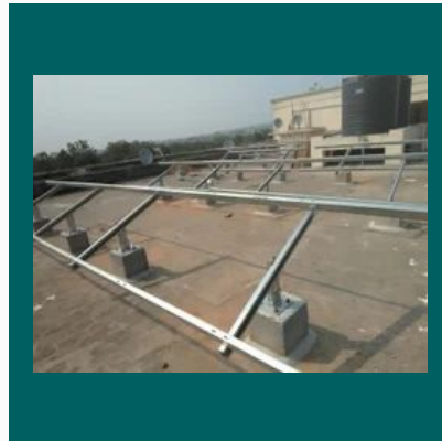
Solar Panel Purlin
