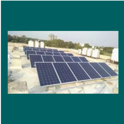
Solar Panel Mounting Structure
