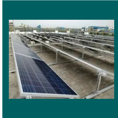
Ballast Type Solar Panel Structure
